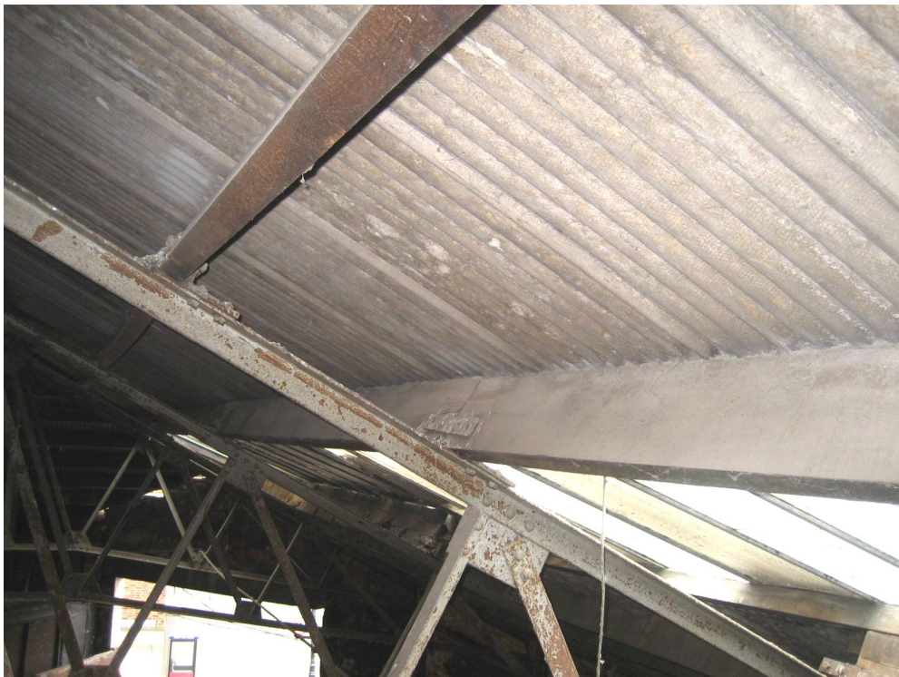
Photograph 46 Purlin connection indicating missing bolts
