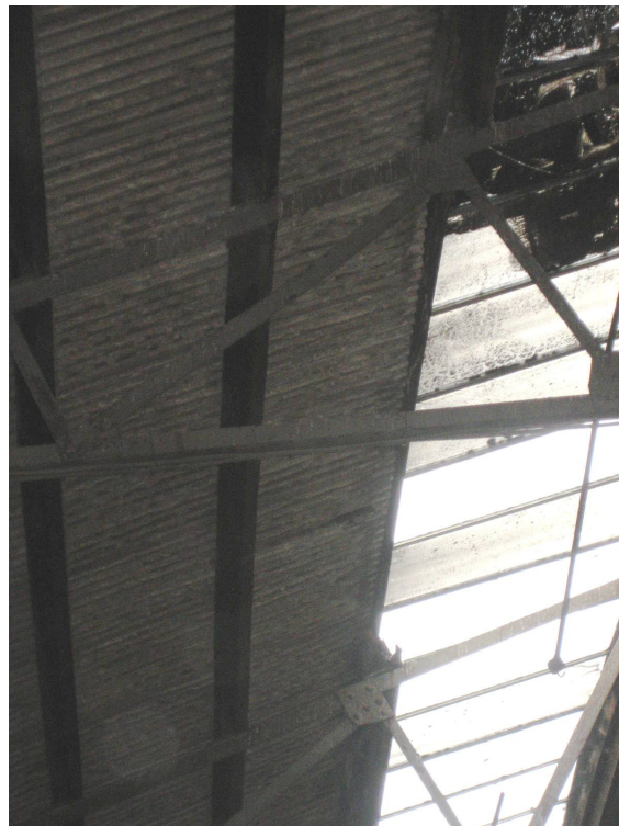
Photograph 34 Missing Purlin in Roof
